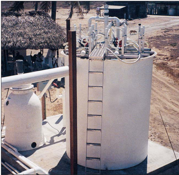
Fluidized-bed biofilter installed in a shrimp maturation system. Photo courtesy of Aquaneering.
